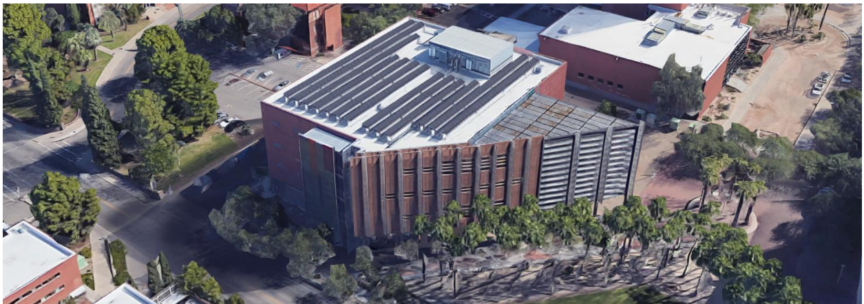
McClelland Park Photovoltaic Installation
